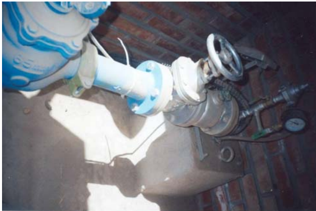
The water system pump at the Elizardo Perez
