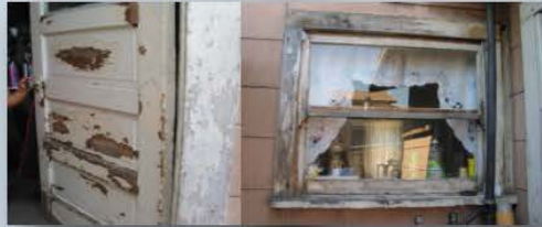
Paint in Homes Built Before 1978
